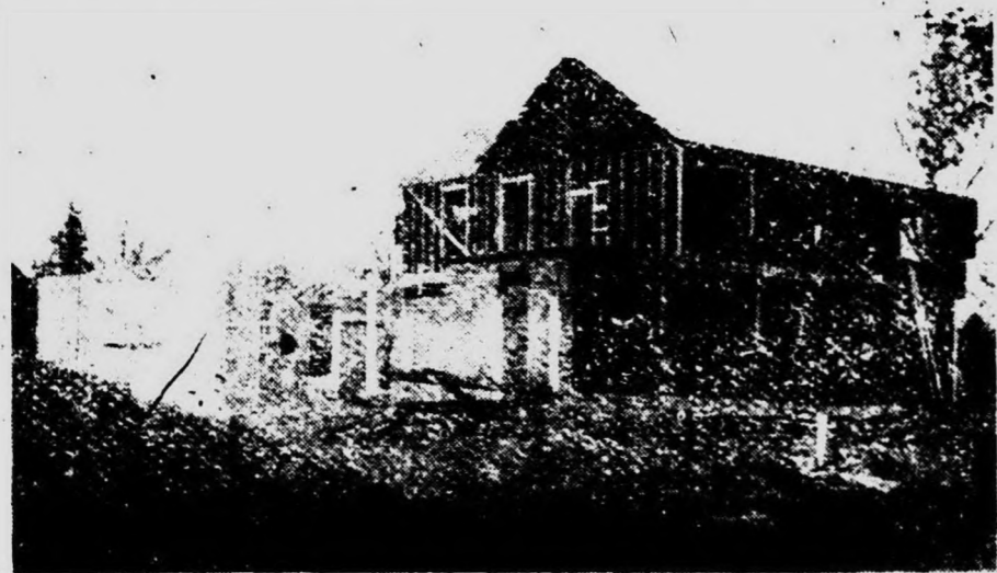
Last of the new homes to be started in the subdivision and probably the largest of the group is the attractive residence pictured here, from the McKinley street side, under construction for Mr. and Mrs. David Mather. The beautiful Mather residence will be the fifth full two story home to be erected in the area, being preceded by the attractive homes of Dr. and Mrs. John Olsaver, Mr. and Mrs. R. M. Daane, Mr. and Mrs. Dow Swope, Mr. and Mrs. Robert Wesley, and Mr. and Mrs. Ciro Scalingi.
