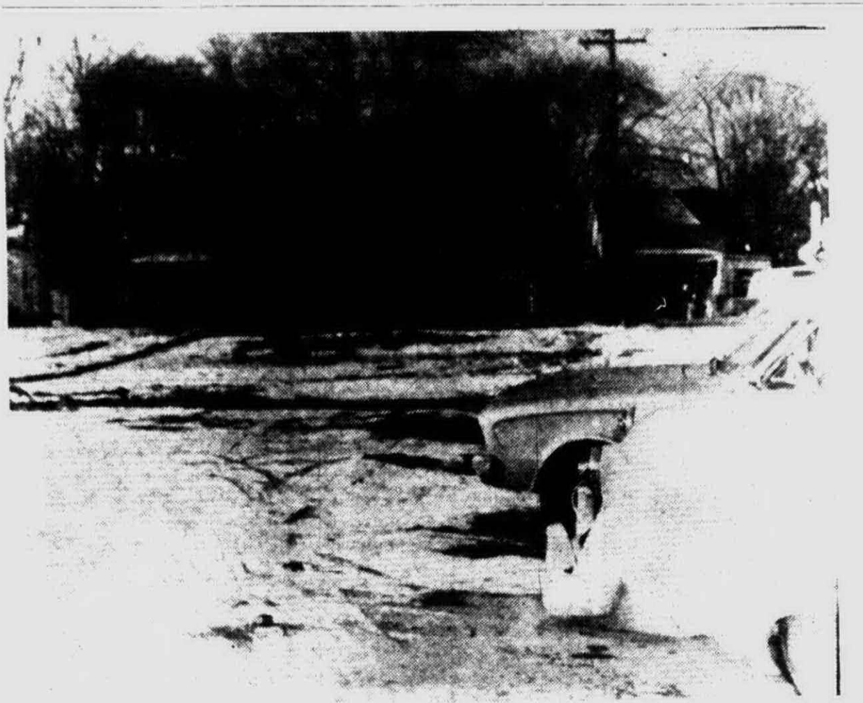
ALL CLEAR AND READY to go. The addition to Plymouth's municipal parking lot will soon be ready for use, with the former buildings which occupied the land completely cleared away. Grading and paving of the lot will soon follow and then it will be ready for auto use.
