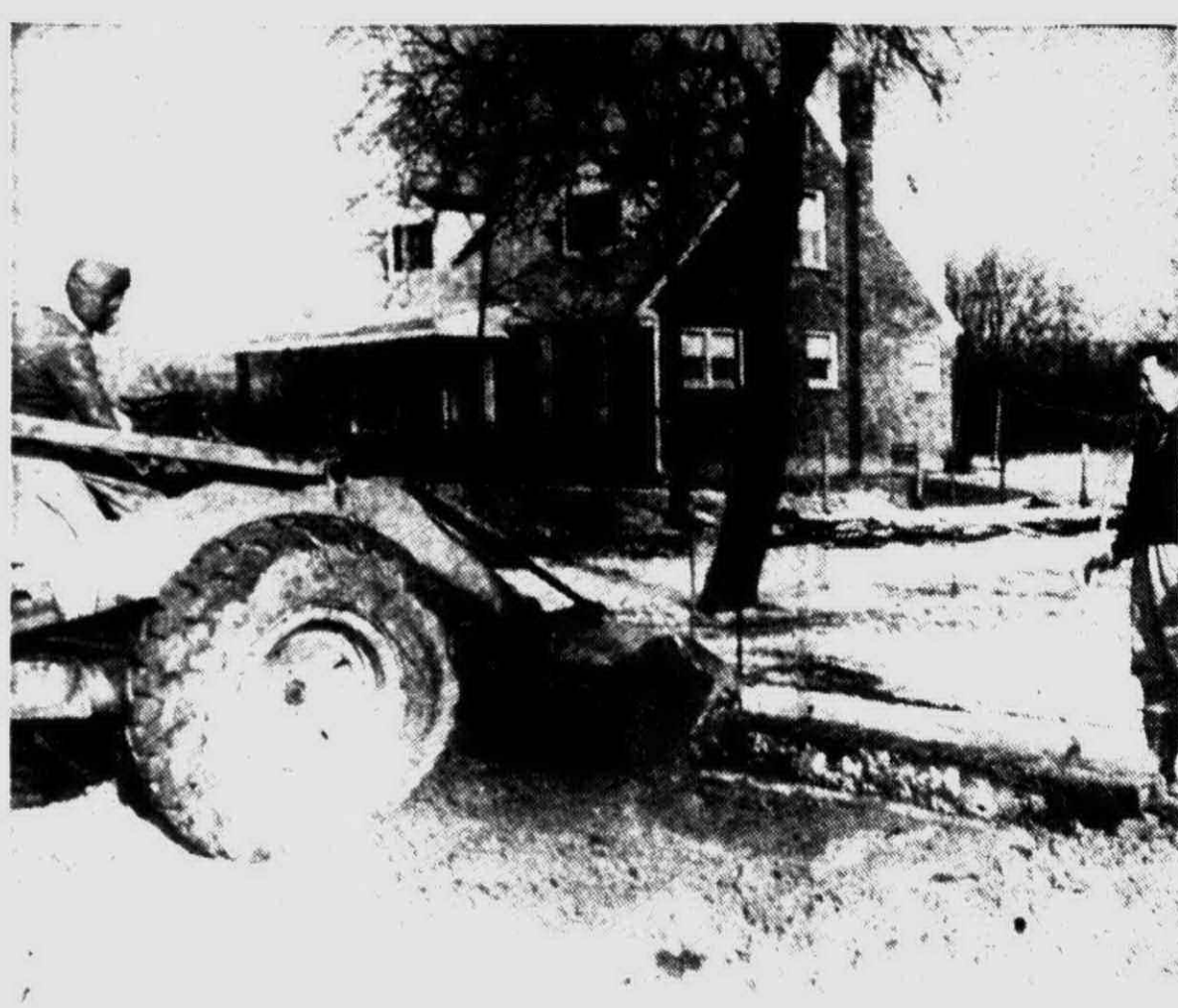
REPAIRMEN WORKED in freezing temperatures Friday to repair a broken water main brought about by near-zero weather. The six-inch break, at Holbrook
