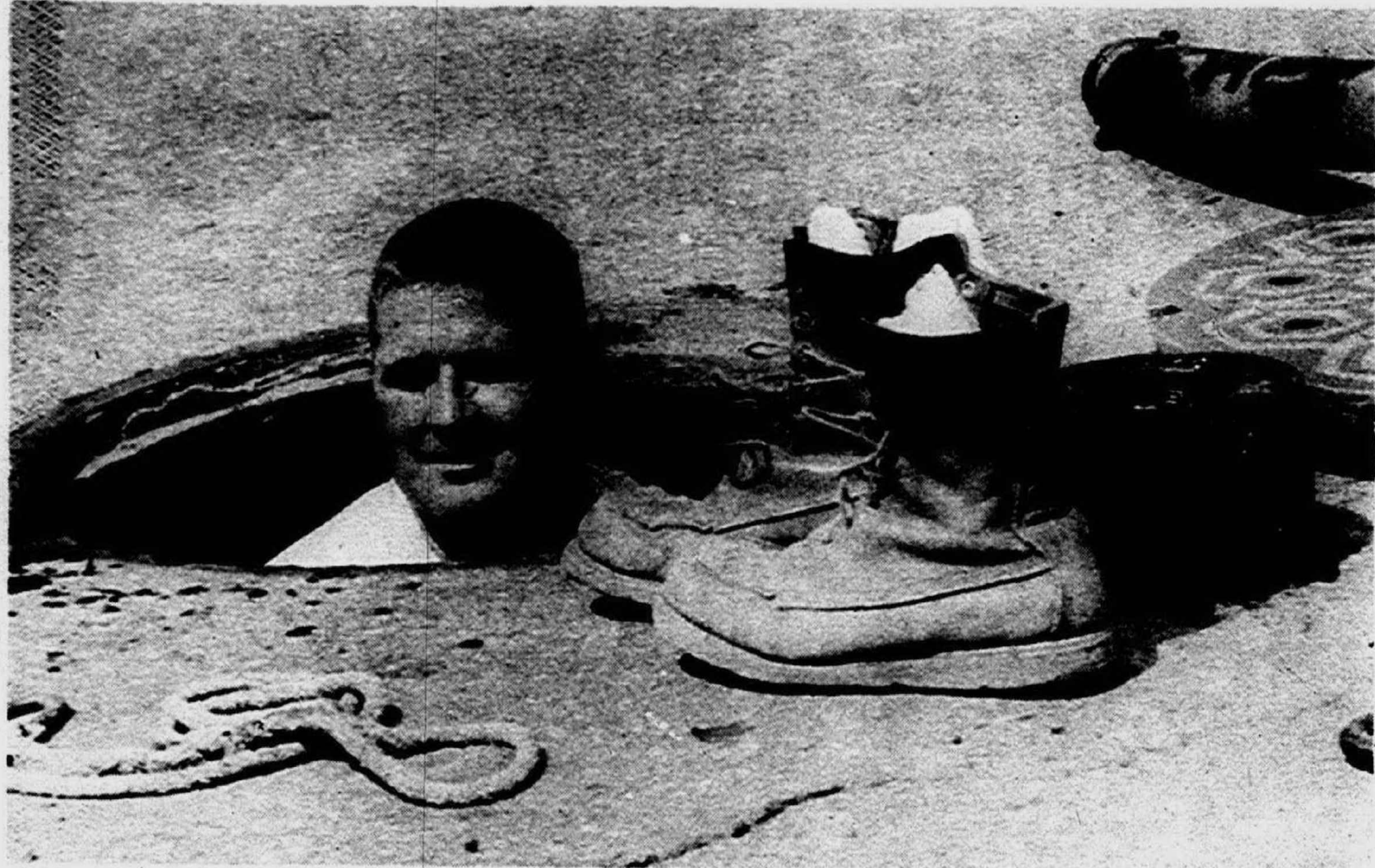
FOR YOUR LISTENING PLEASURE: There is a lot more to a telephone conversation than picking up a phone and starting to talk. There are miles and miles of wires underground and they are
