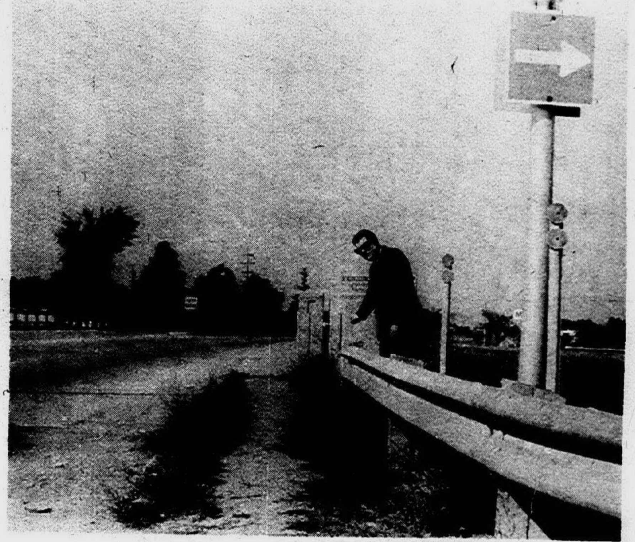
"Here's a glaring example of misuse of a guard rail. A driver going off the road would be forced by the rail into this concrete abutment. The rail should go out to the front of the abutment, not into the side." Scene: I-96 in Farmington.
