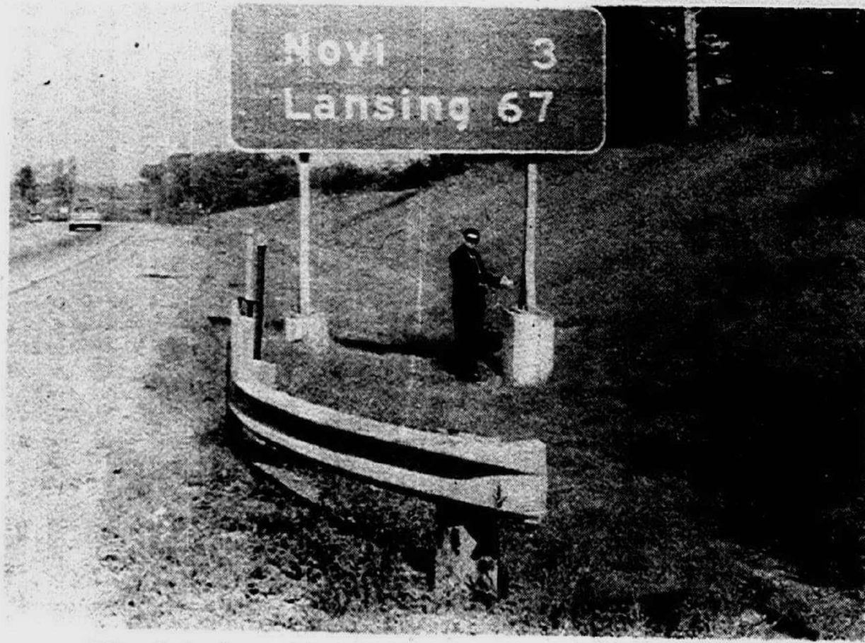
"Two faults here. First, here's a sign within a few feet of the roadway. The sign is embedded in concrete, and this type of sign costs about $2,000. A break-away sign would be cheaper, or the sign should be well off the road. Second, a rail had to be put up to protect the sign—not the motorist. The front of the guard rail (toward camera) has a knife-edge. It should be flared and the edge buried. I have a picture in Washington, D.C., where over 75 feet of this kind of rail have gone into a car." Scene: I-96 in Farmington.
