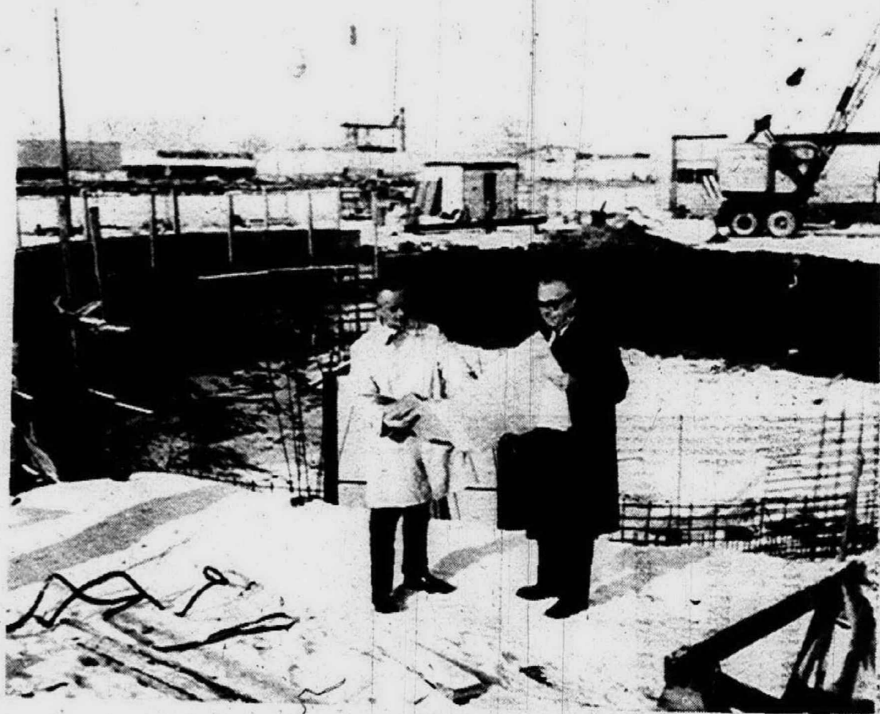
CHEVROLET SPRING AND BUMPER PLANT MANAGER, Harrison T. Price, (left), and Fisher Body plant manager, F. Harger Green make year-end check on construction progress of Chevrolet's new storm water separator system. Designed solely to help protect the purity and wildlife of Newburgh Lake, the 330,000-gallon clarifier tank will eliminate most of the oil and other waste materials washed into the sewer from the plant site by heavy rains.
