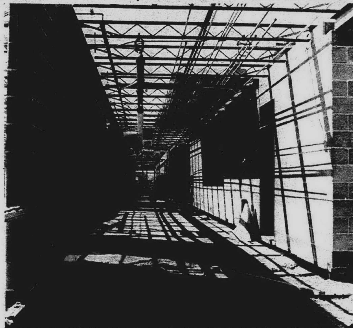
PLYMOUTH'S MIDDLE SCHOOL No. 3, on Ann Arbor Rd., is ready for bricklayers, but they're on strike and may be for a long time. Six unions are on strike against the association of contractors.
