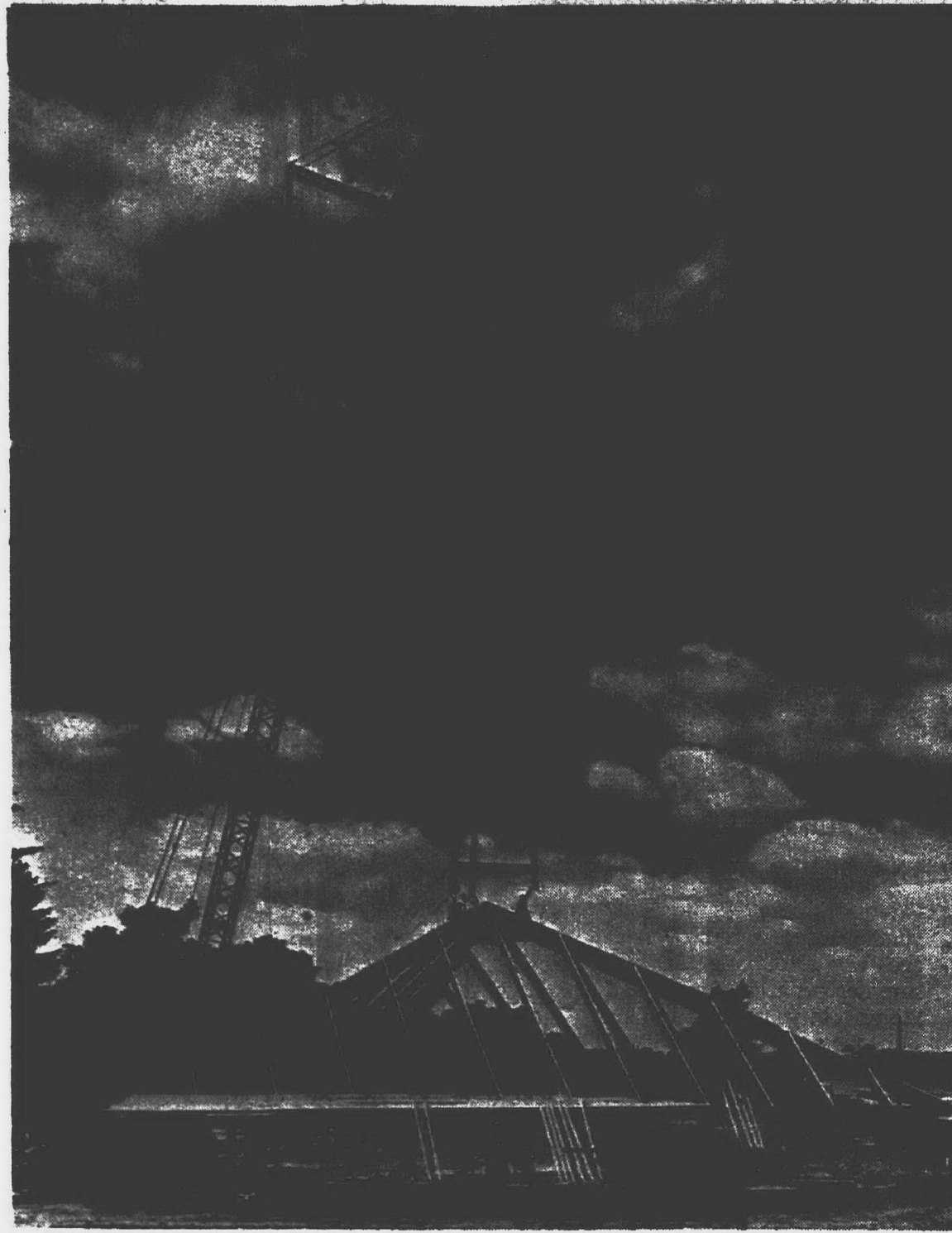
A STEEL TOWER that is bound to become a landmark in Farmington was lifted into place atop the frame of the new University Hills Church at Farmington Road and the I-696 Freeway last week. The tower weighs 6 1/2 tons and will rise 165 feet into the air. It was assembled on the ground before the huge crane gently lowered it to the peak of the triangular-shaped church building. The church, being constructed by C.H. Haberkorn & Co., Orchard Lake general contractor, is due for completion in mid-October.
