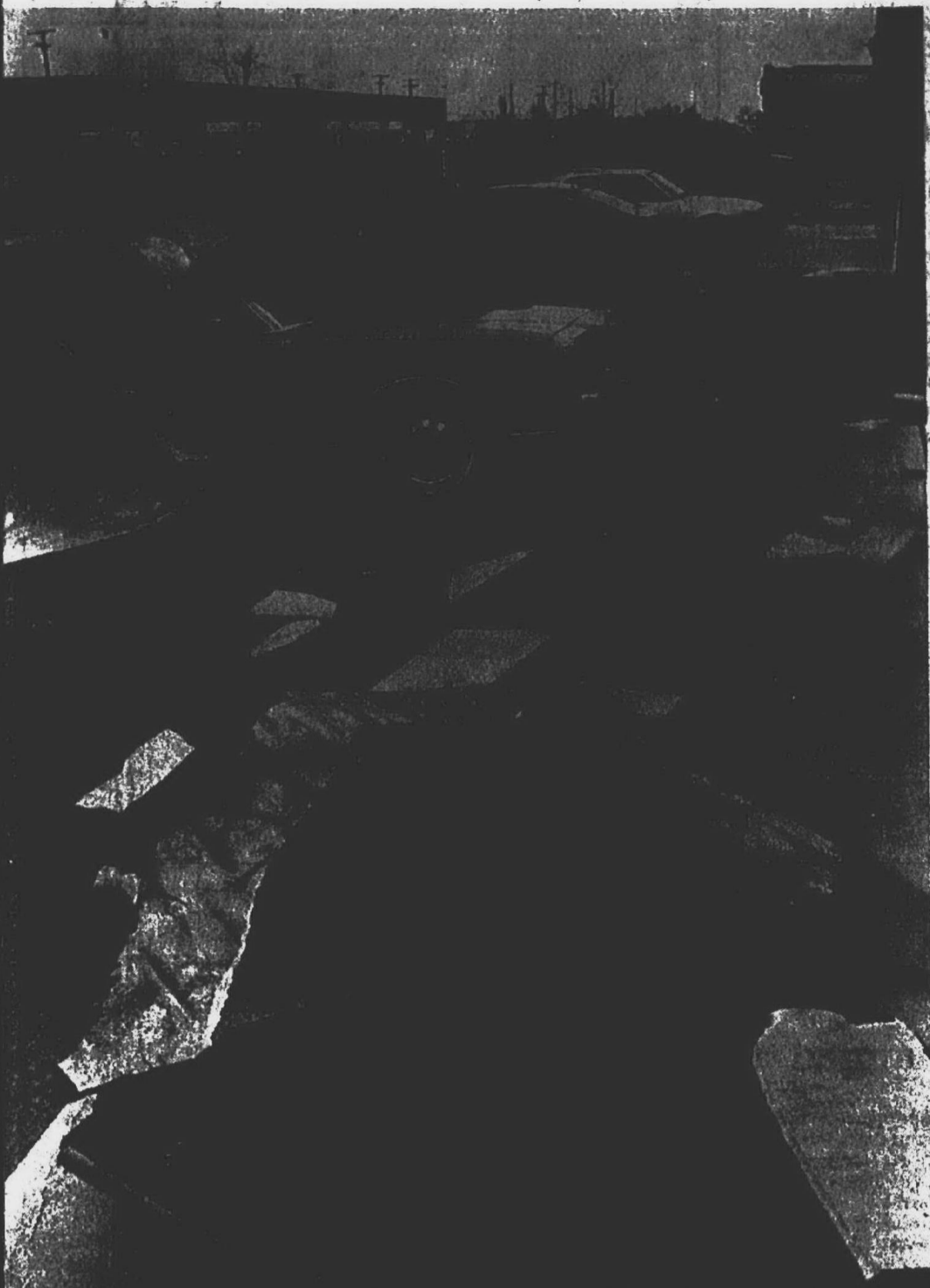
High winds caused the roof to blow off a row of offices on Joy Road next to Mettetal Airport in Canton. The large pieces of
