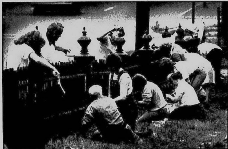
'Project Ginny' participants had to wire brush the rusted areas of the Redford Township Pioneer Cemetery fence on Telegraph Road before painting it.
