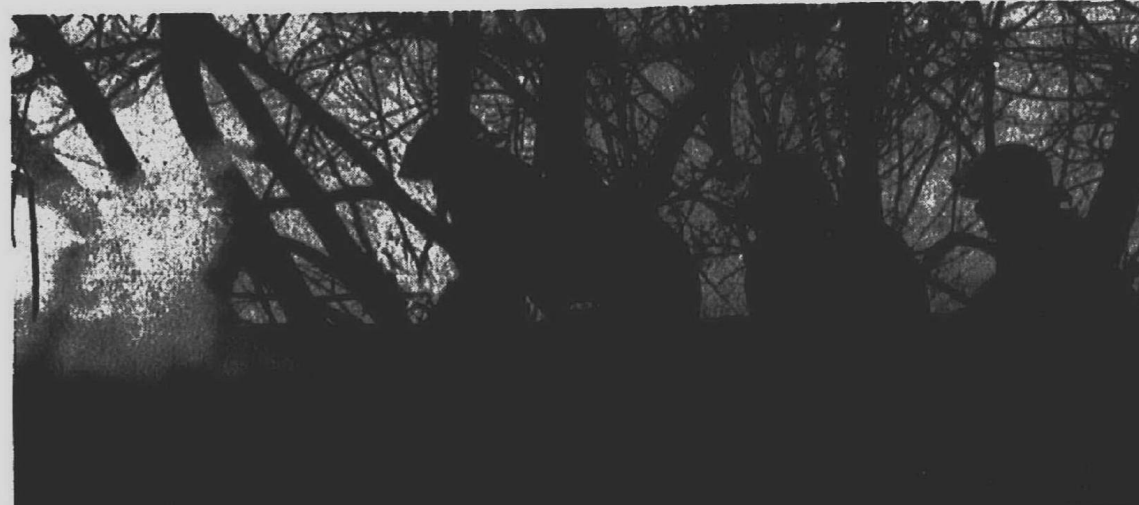
Firefighters chop a hole in the roof to ventilate smoke and gases.
