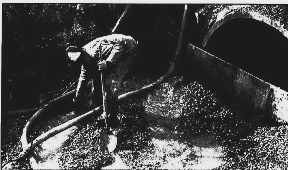
One would expect to find water in a drainage ditch but, in this case, the flow slowed down construction over the weekend on enclosing the Tonquish Creek. A worker is shown here Saturday pumping water.
