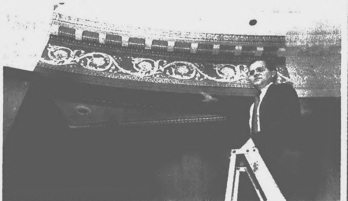
Paul Ganson climbed a ladder to call attention to the look of the newly restored cornice.
