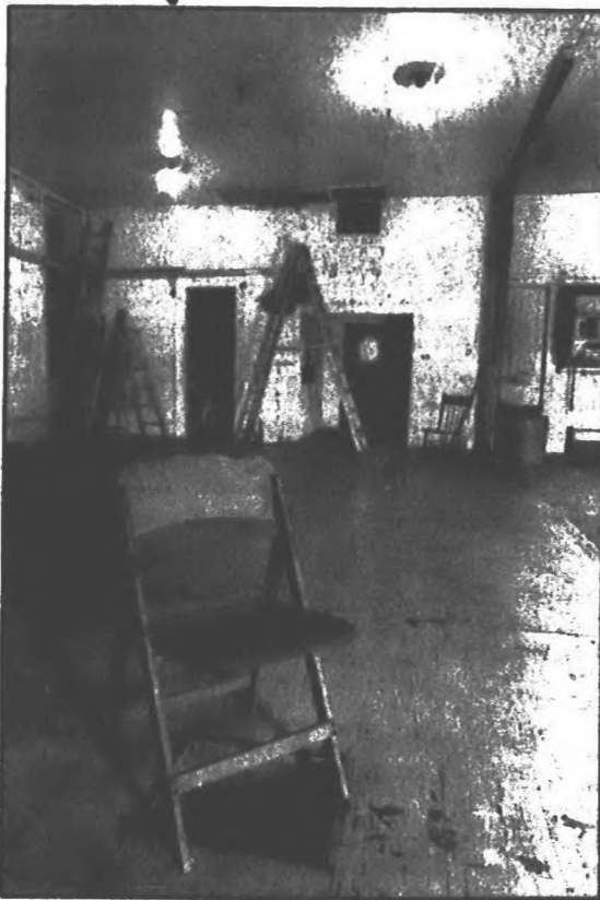
The interior of the school house is nearly gutted.
