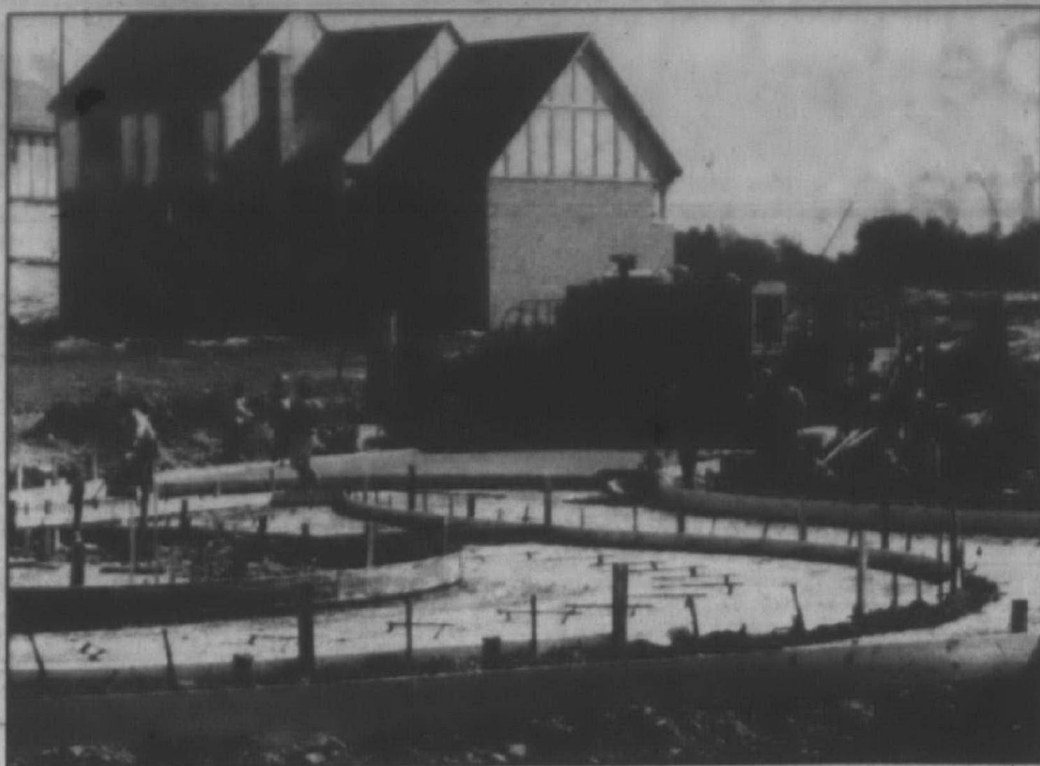
A concrete hauler's strike has put a damper on construction projects from the laying of curbs to the pouring of foundations.
