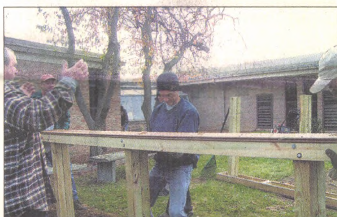
From left, Doug Linsenmann, Paul Bingham, Phil Pairitz and Barry Bridges work on installing one of three 12-foot benches in a courtyard at Pioneer Middle School. Boy Scout Steven Cadwell enlisted help from around 40 people, some 30 fellow scouts and around 10 parents, to give the courtyard a facelift on Oct. 29; the project was one of the steps required as Steven works toward an Eagle Scout rank.
