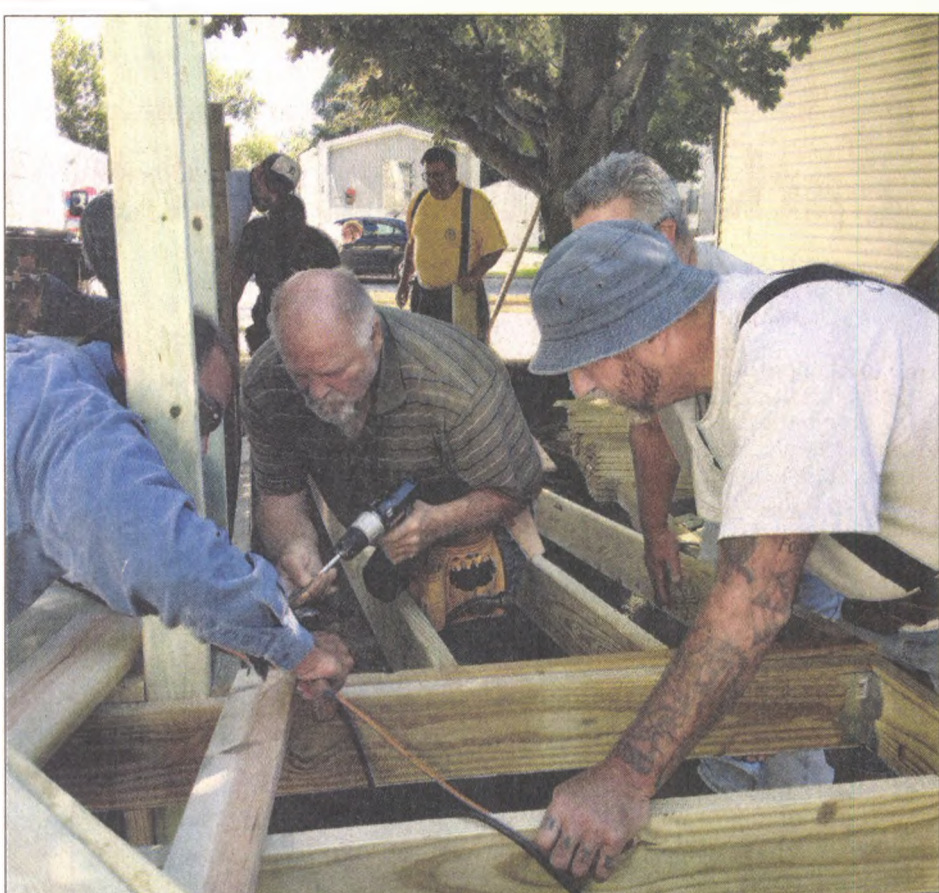
Volunteers from a variety of locals of the Michigan Regional Council of Carpenters and Millwrights helped put a ramp and a new deck on the home of a retired union member from Canton.
