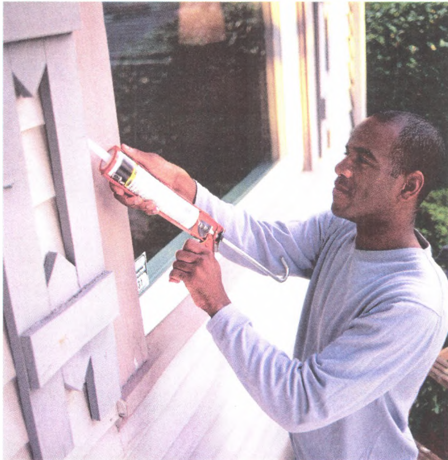
Use caulk or concrete to repair all cracks, crevices and leaks no matter how small. GETTY IMAGES | FUSE
