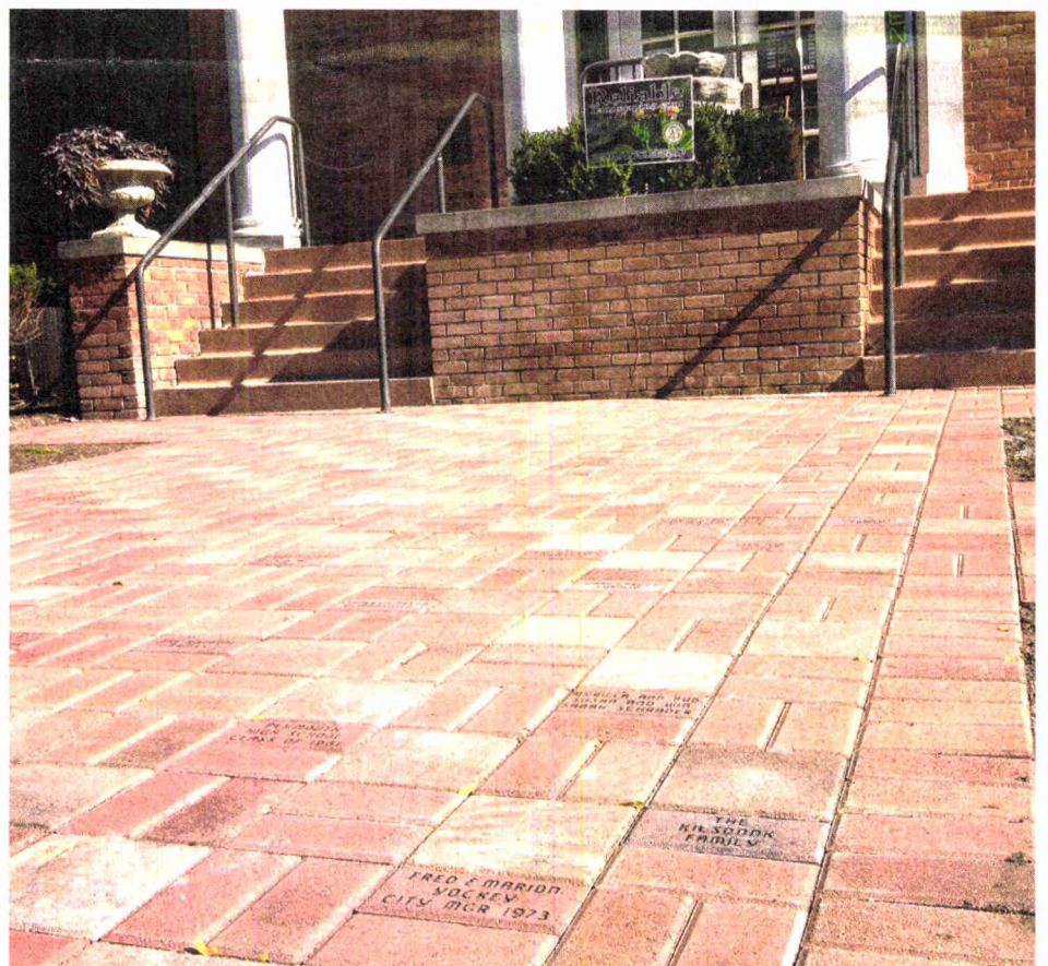
The Plymouth Historical Museum’s new brick-paver patio was installed in front of the building Tuesday. There are about 90 dedicated, engraved bricks in the patio and more will be added, in batches, as they are purchased.
